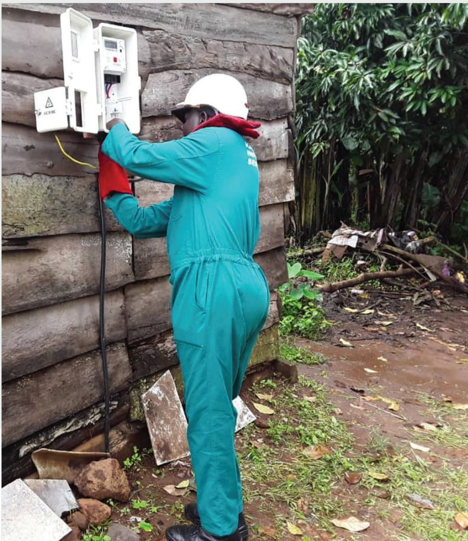
A wireman installs an electricity connection on a residence. Photo: Barnabas Mugabi/Power Africa Uganda Accelerator.
